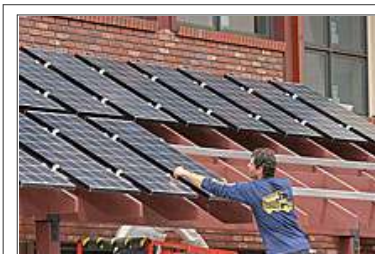
Ilan Levy, working with SunJuice Solar, installs photovoltaic solar panels on the Sundance Professional Centre, a medical office building on the northeast corner of North Lincoln Avenue and West 29th Street. The solar power system will be the first in Loveland to connect to the city's utility grid and has prompted city utility officials to propose policy changes to accommodate the increasing popularity of renewable energy. Reporter-Herald/Heather A. Longway-Burke
